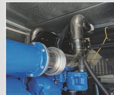
Interior of the genset
